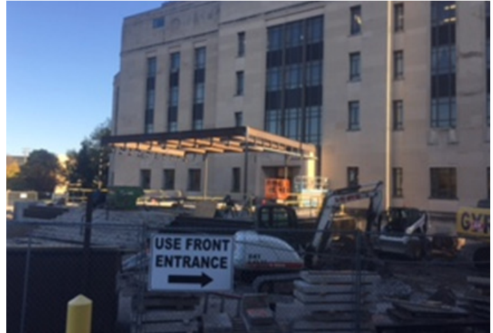
A new security checkpoint is among projects being undertaken at the Winnebago County Courthouse. Other improvements include construction of a dedicated room where suspects can be processed.
