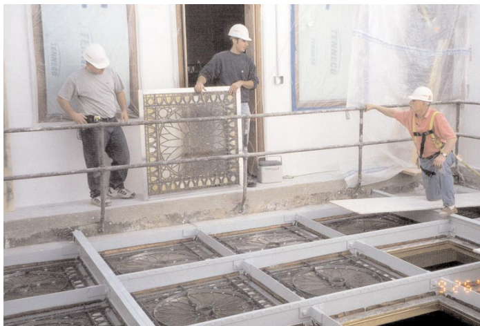
Workers carefully removed the skylight in the Supreme Court Hearing Room as part of the restoration process.
